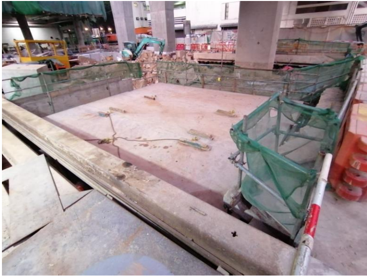
Figure B3: Closure of Acoustic Panel
