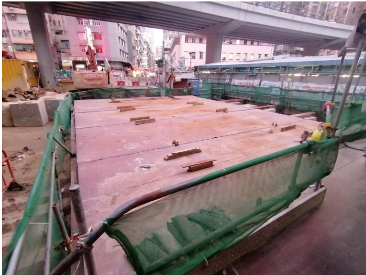
Figure B4: Closure of Acoustic Panel
